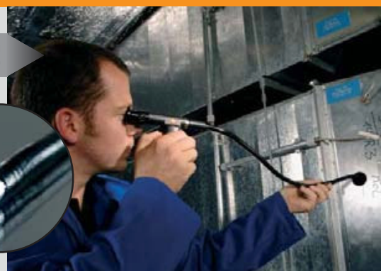
Inspects air duct, with gooseneck casing, middle flexibility
