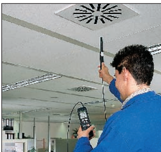
Measures CO2 concentration in ingoing and outgoing air ducts
