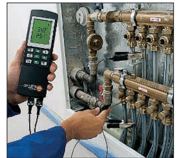
Fine adjustment of the flow and return temperature in floor heating using a clamp probe
