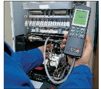
Adjustment of gas flow pressure in a gas heater (adjustment values in natural gas: 20-25 mbar)
