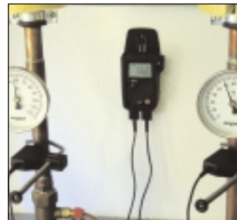
Checks flow/return temperature in heating systems
